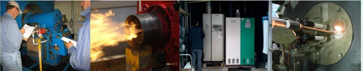
CFE Plant in Mexico Auxiliary Combustion E-80M
